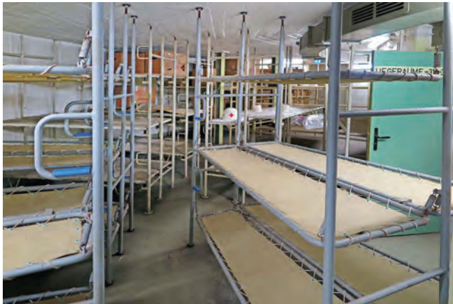
Dormitory within the Berliner Tor bunker. The three-level bunks are packed into the available space but it can be seen are jammed rather than firmly fixed into the structure to minimise the effect of blast
